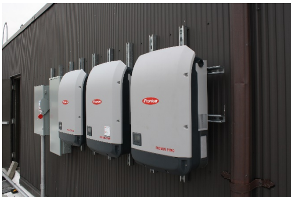
Bank of String Inverters
